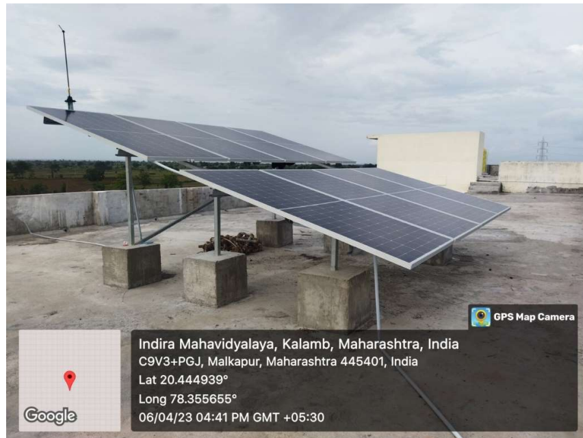
4.0 KW Rooftop Renewable Energy Generating System for Consumer
